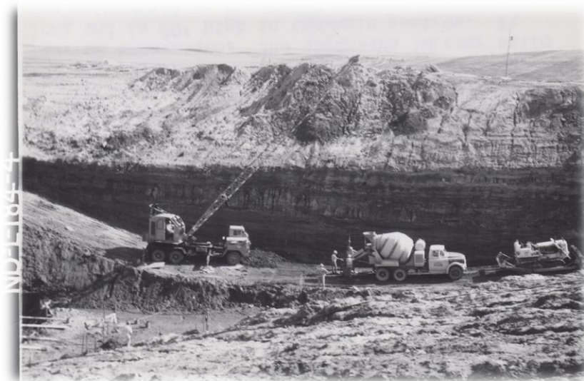
Figure 31. Construction of the north side of the spillway of the Bowman-Haley Dam.
